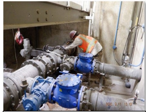
Delta Diablo Pump Station Piping
