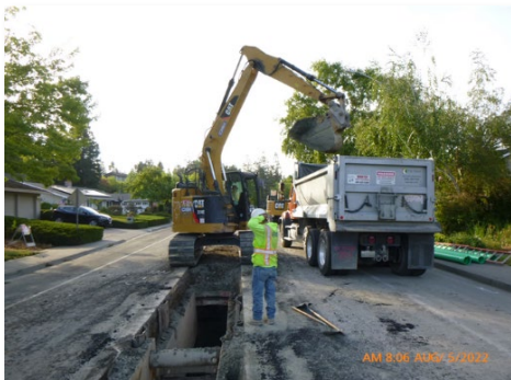
Central San Sewer Pipeline in Road
