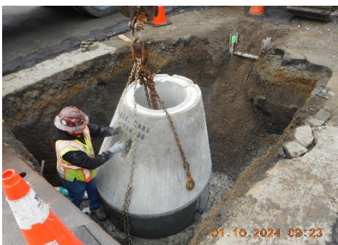
Central San New Sewer Manhole
