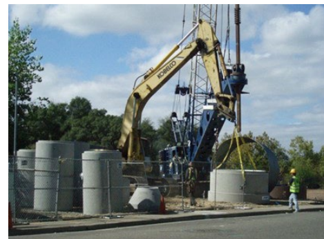
Lake Forest Pump Station Wet Wells
